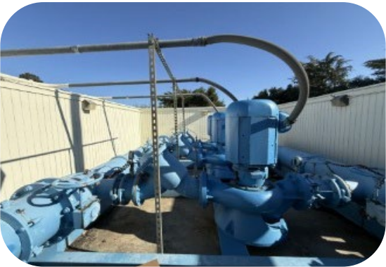
Silver Oaks Pump Station
