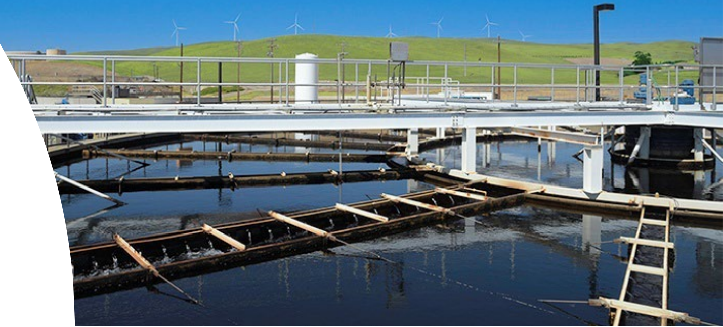
Clarifier at Patterson Pass Water Treatment Plant
