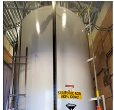
New Chemical Storage Tank at the Mocho Groundwater Demineralization Plant
